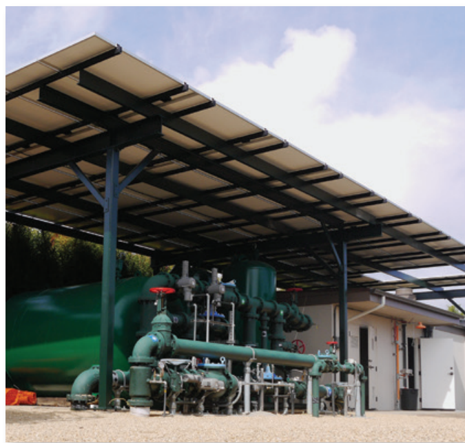
The District is tapping into its diverse groundwater supplies with state of the industry technologies.
