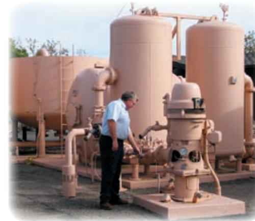
Newly refurbished groundwater wells and pump facilities. The District has not used any groundwater for over ten years, saving it for future need.
